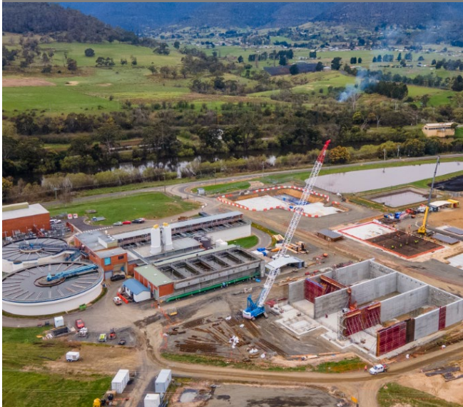
Bryn Estyn Water Treatment Plant
